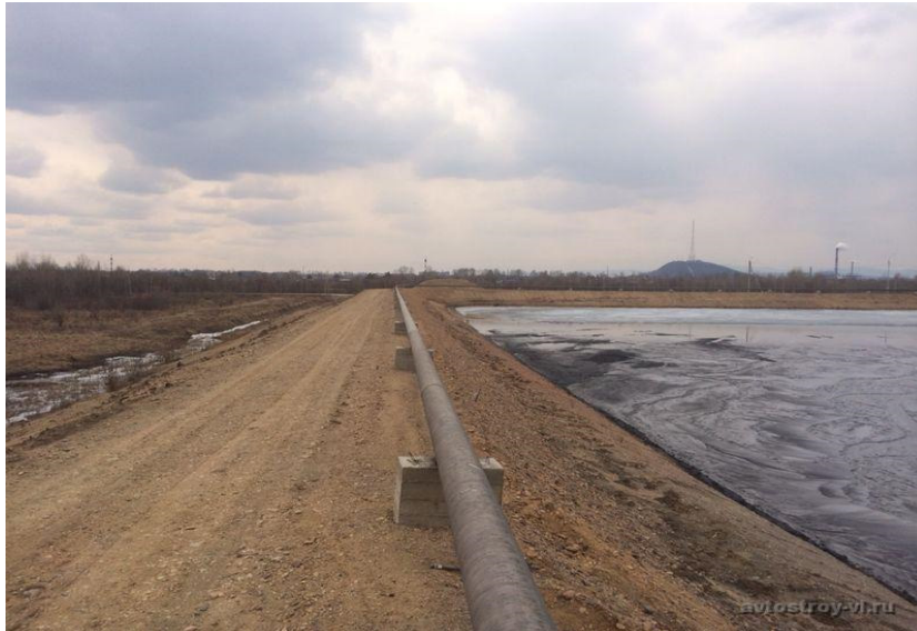
Figure 2. Bulk embankment No. 1 of the ash dump of Topar Main Distribution Power Station LLP.
