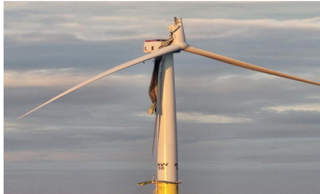
Figure 4. Photographic evidence of the Dogger Bank wind turbine blade damage [51] .
