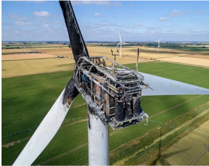
Figure 4. Consequences of a fire in the turbine nacelle – a destroyed nacelle on a V150-4.2MW Vestas turbine at the 164MW Myrnenska wind farm in Ukraine [7] .
